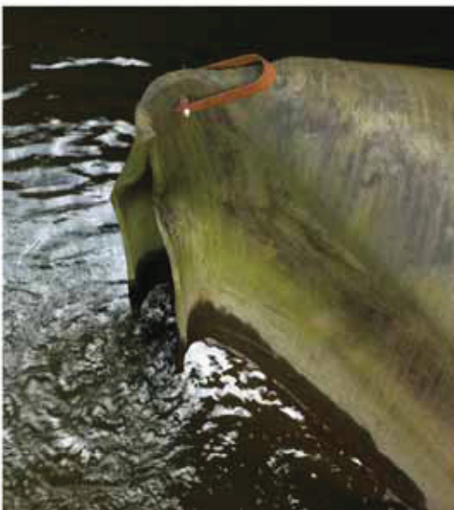
Destroyed Curved Bill Style Check Valve
