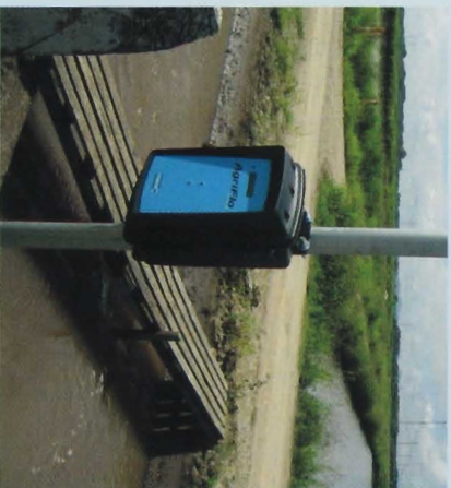
Figure 2: A Series3 Agriflo installed on the delivery channel of the Costa Rican Tilapia farm.
