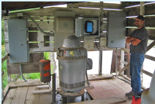
Figure 2: One of twelve MACE AgriFlo units installed along the Sacramento River in Northern California.
