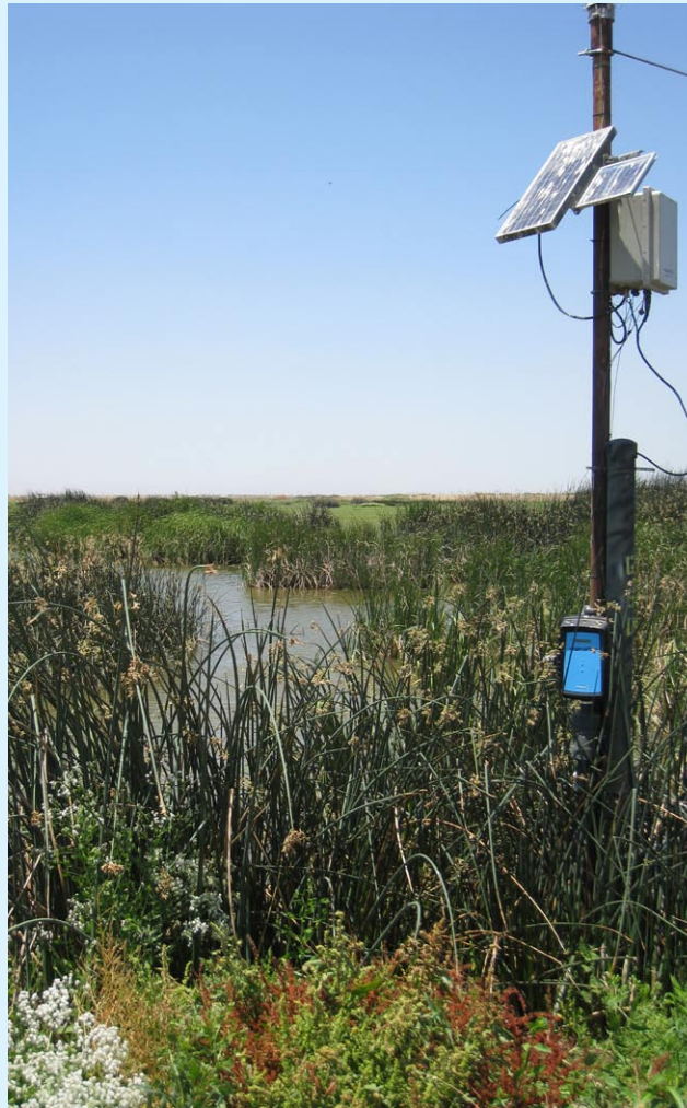
Figure 3: A Series3 AgriFlo installed on the outlet of a lagoon.
