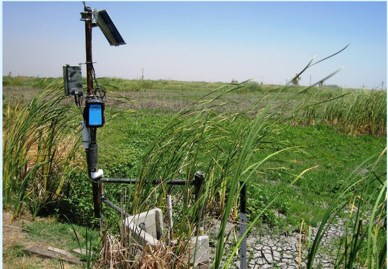
Figure 1: An outlet of a pond near Los Banos, CA. Note the headwall of the 18" pipe.
