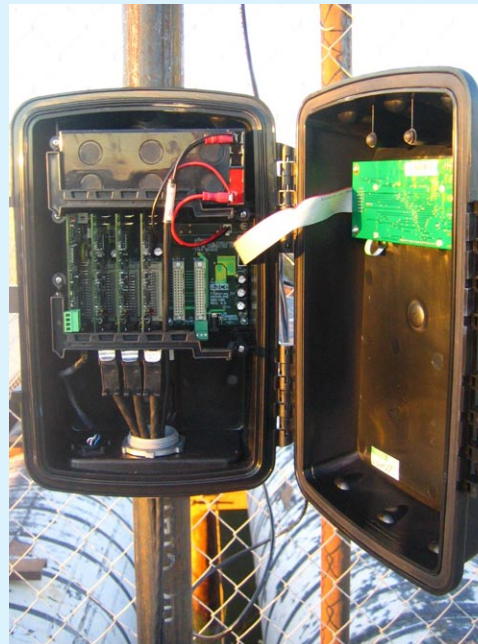
Figure 4: The Series3 MACE AgriFlo unit installed on Quail Mesa Ranch. Note the 3 sensor cables entering the AgriFlo enclosure.
