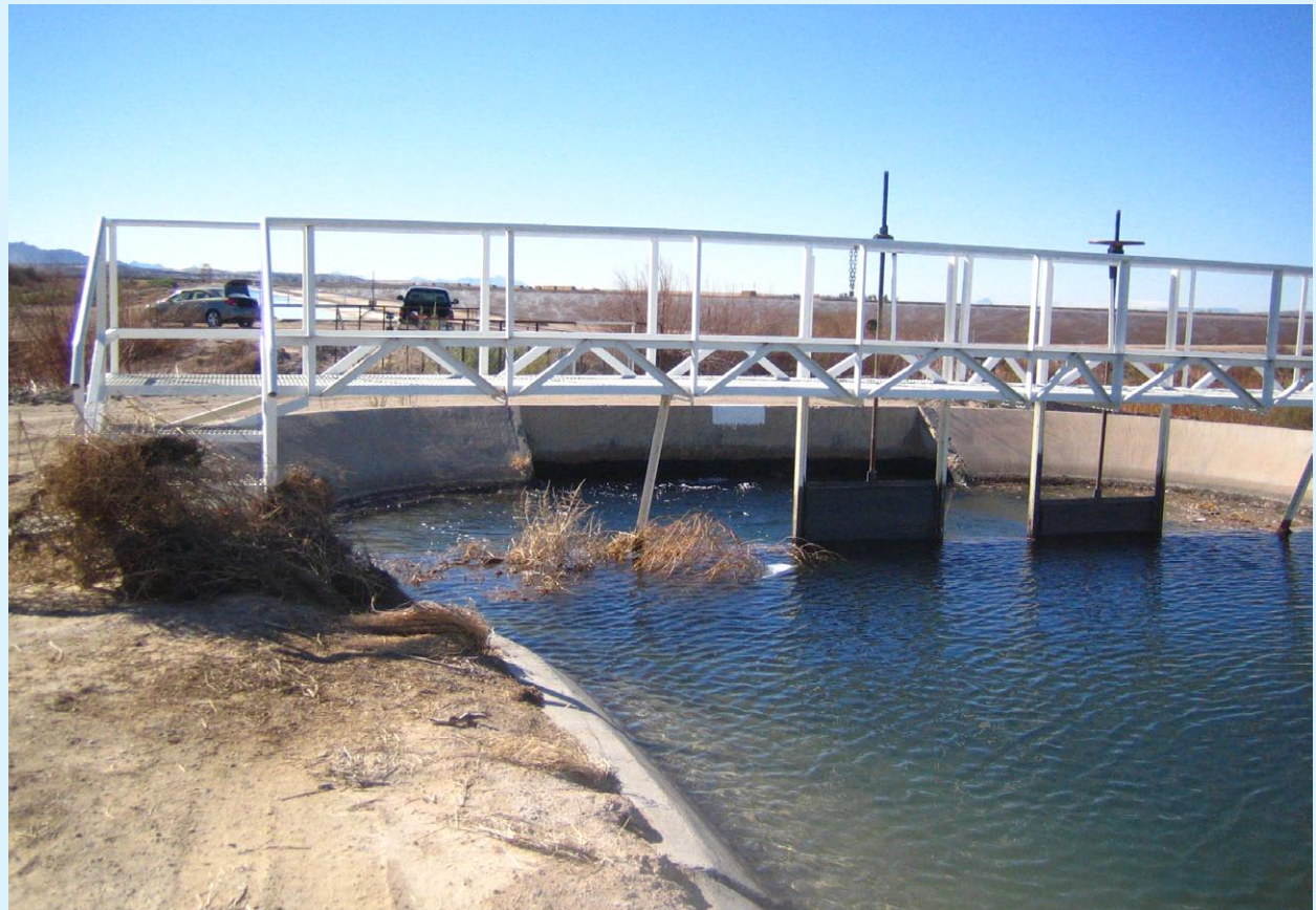
Figure 1: The outlet of the large USBR supply canal at Quail Mesa Ranch, AZ.
