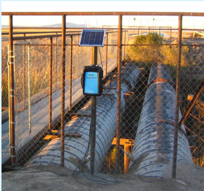
Figure 3: The Series3 MACE AgriFlo unit installed on Quail Mesa Ranch. A 2" insertion sensor is installed in each of the three 47" pipes.
