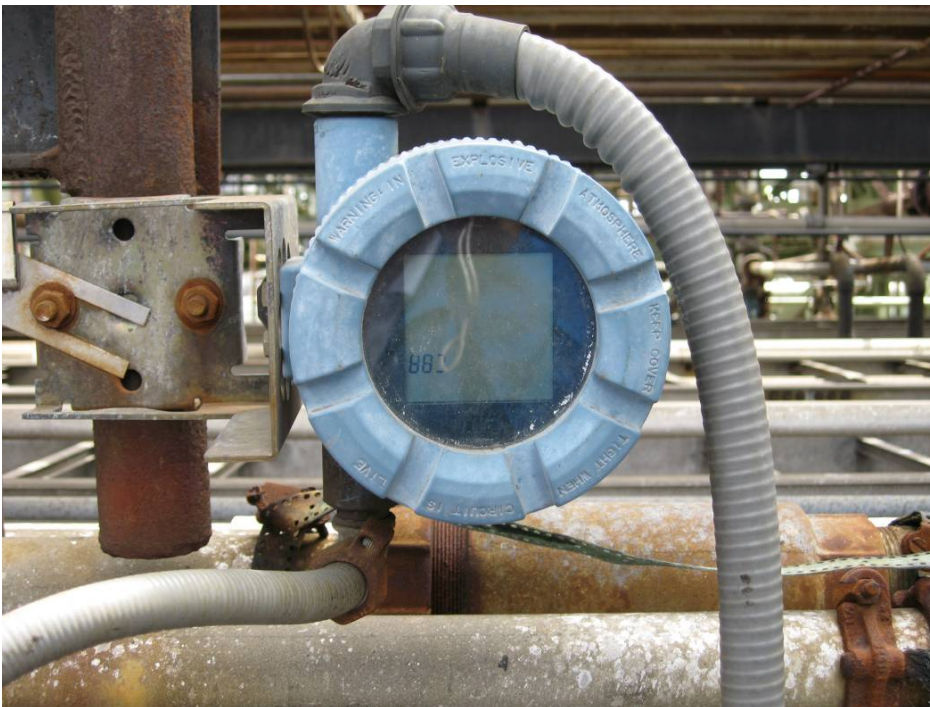
Failed new technology transmitter, recommend replacement with Stratos
