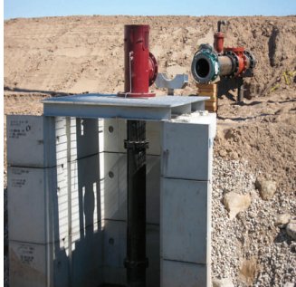
Vertical pump to transfer seepage from second canal to primary canal
