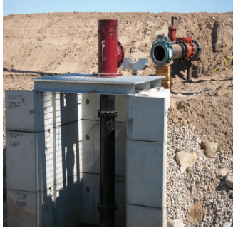
Vertical pump to transfer seepage from second canal to primary canal
